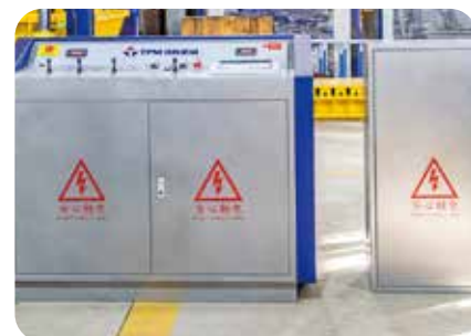
Siemens PLC Control System and Siemens Remote Control System
