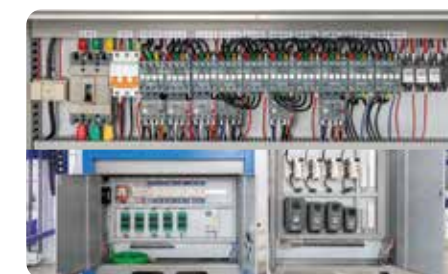
8. Separation of the strong current and weak current in the complete electrical control system, to avoid mutual interference. Online troubleshooting through internet to achieve the future program update and remote fault diagnosis.
