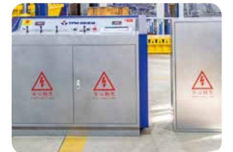
Siemens PLC Control System and Siemens Remote Control System
